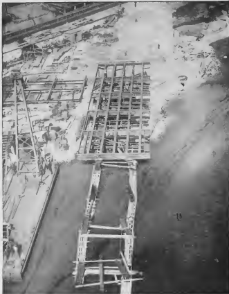
The new No. 1 (East) Finger Pier, now under construction, will be one of the largest all-welded steel oil-handling piers in the world. It will reach 790 feet from tip to shere, and will berth two 26,000 ton ocean tankers.
